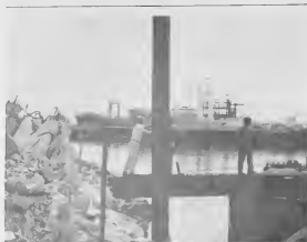
THE FIRST pile of the new No. 3 Finger Pier stands in place ready to be driven into the ground. The pile is held in place by a steel pipe and bracket extending off the crane barge.
